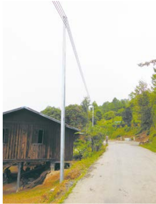
Fig. 10. Newly installed post for power supply in Kanpetlet. Also note a typical house with stilts (April 2016).
