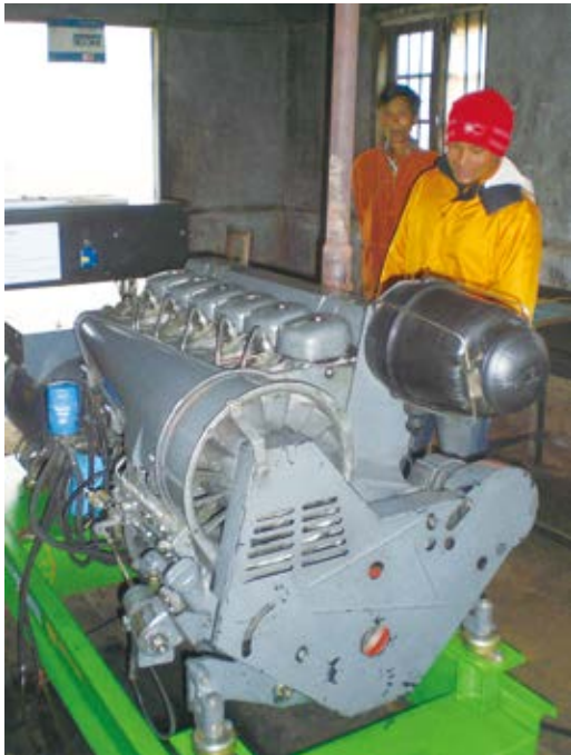
Fig. 9. The diesel generator at the power plant in Kanpetlet (November 2008).
